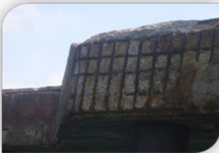
Spalling concrete wharf structure
